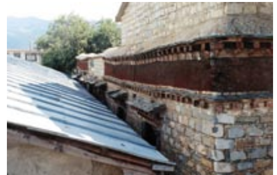
The east elevation was permanently blocked in the 1970s by the construction of a corrugated-iron storage hall (1996 AA).
