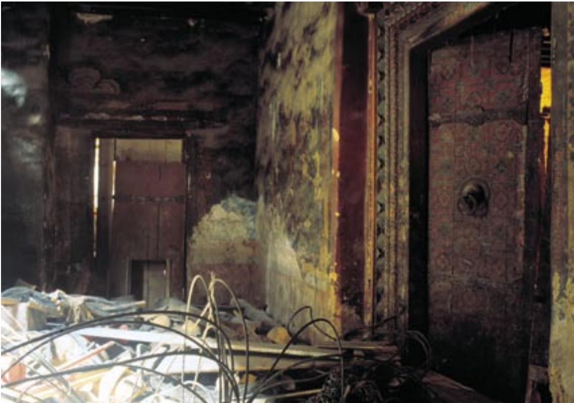
The ambulatory passage is no longer in use and is littered with garbage; the western portion is shown here (1996 AA).
