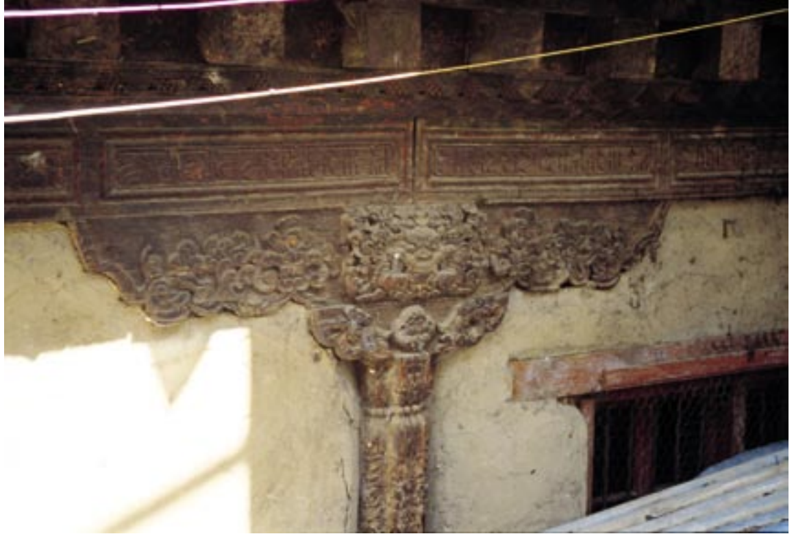
Detail of the portico timber frame; an exceptionally well-carved dzibar image adorns the pillar capital (1995 AA).
