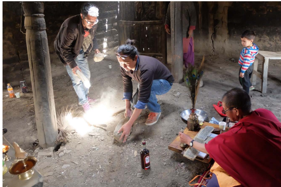
In the summer kitchen on the top floor of the Kushu house, architect Yutaka Hirako (centre) participates in a religious ceremony before commencing repair work.
