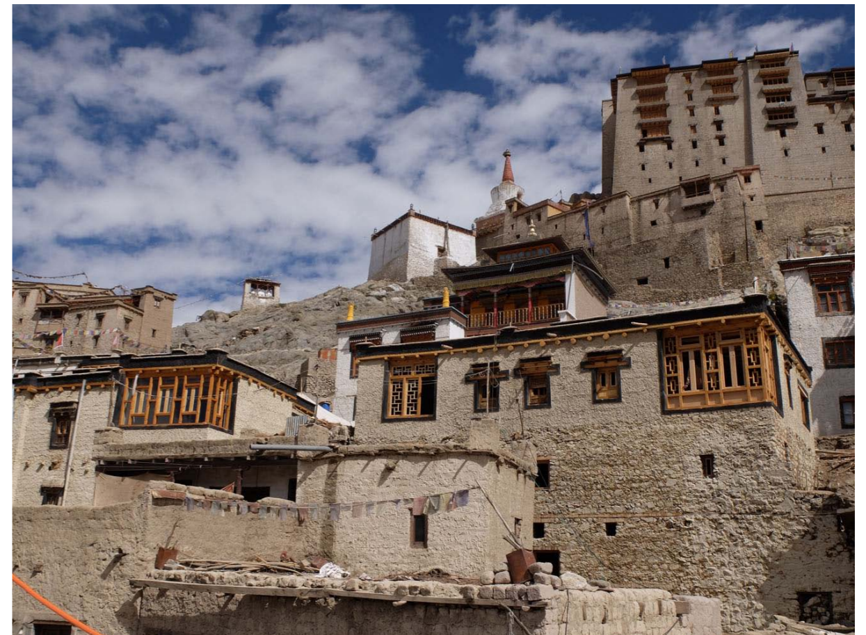
The Kushu (left) and Dzomskit houses after repair, with the Leh palace in the background
