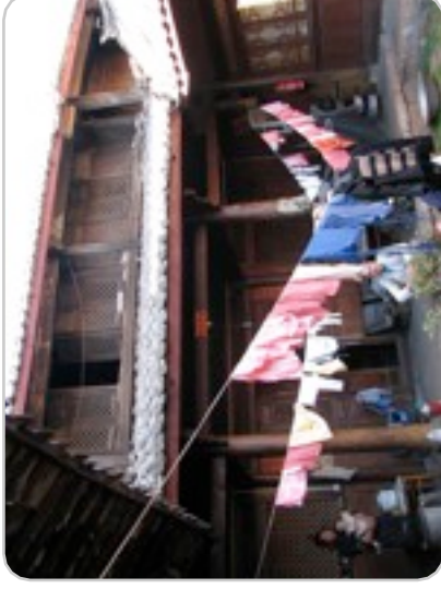
Verandah of low-income, whose house was partly repaired by the government.
