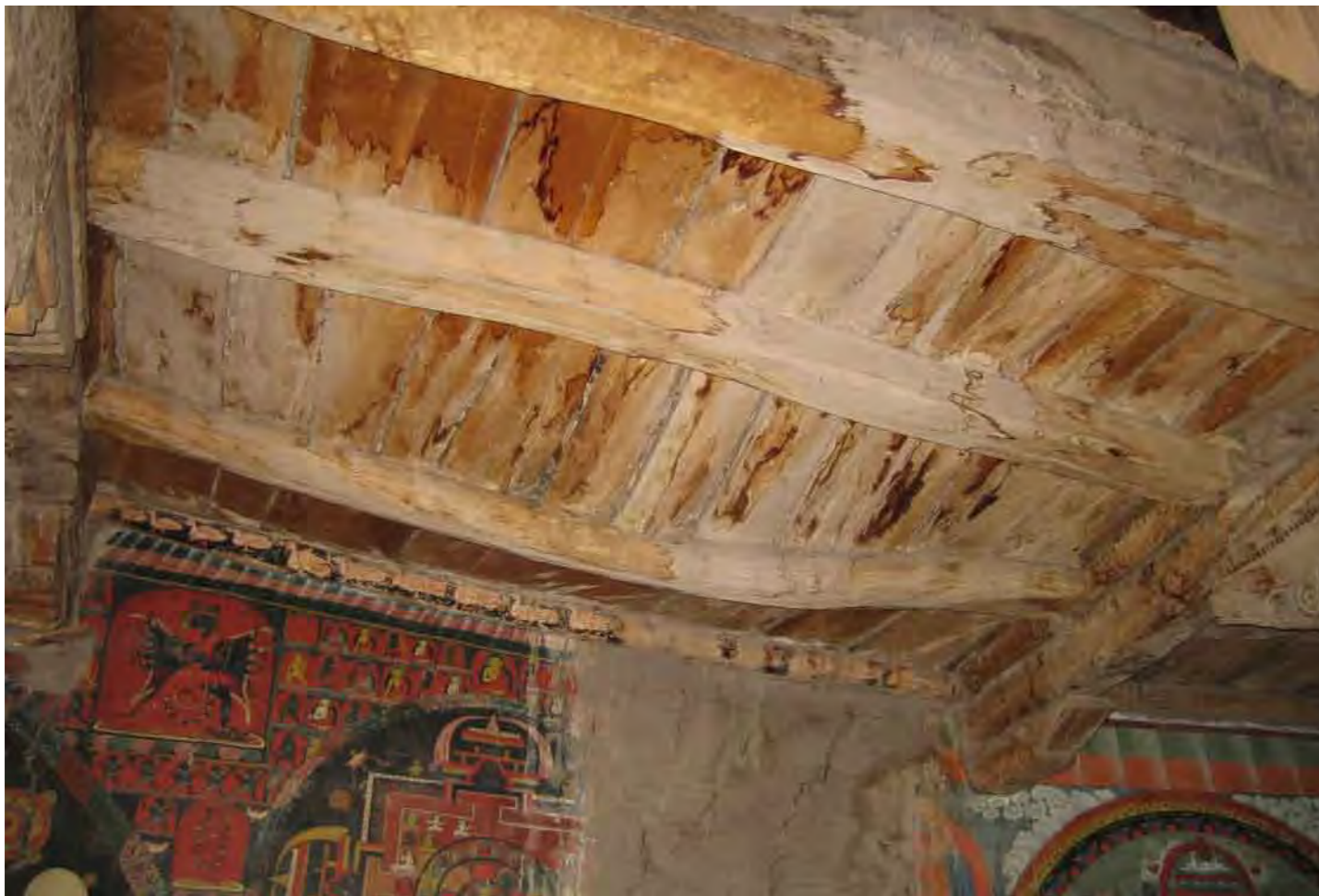
Dukhang 1st floor - damages at ceiling and walls caused by roof leaks
