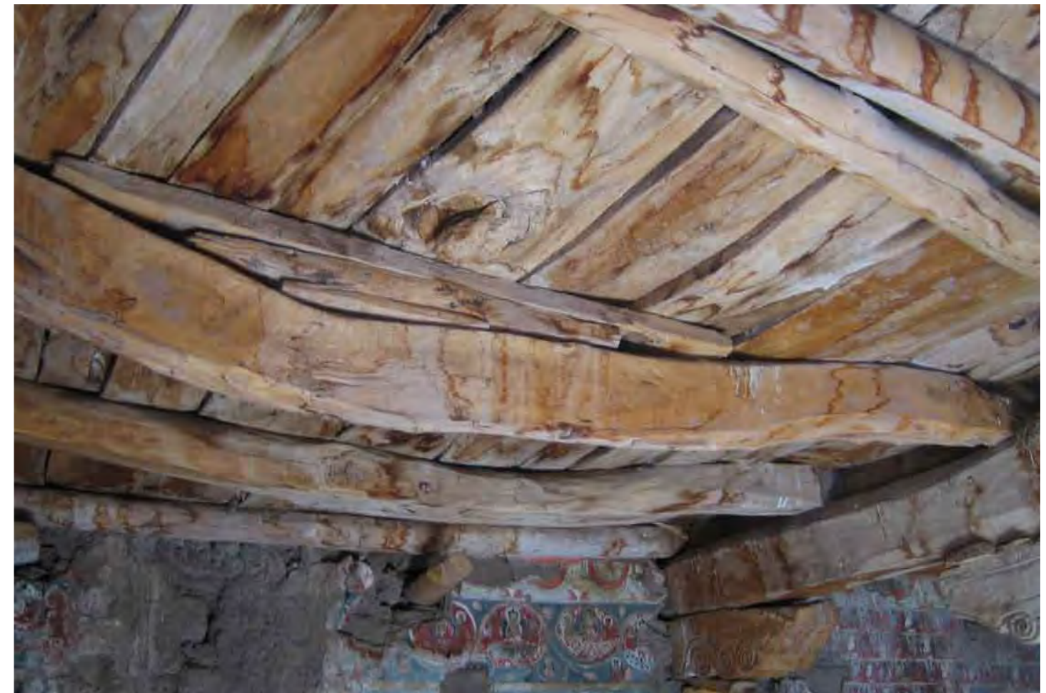
Dukhang 2nd floor - deformation of load-bearing elements
