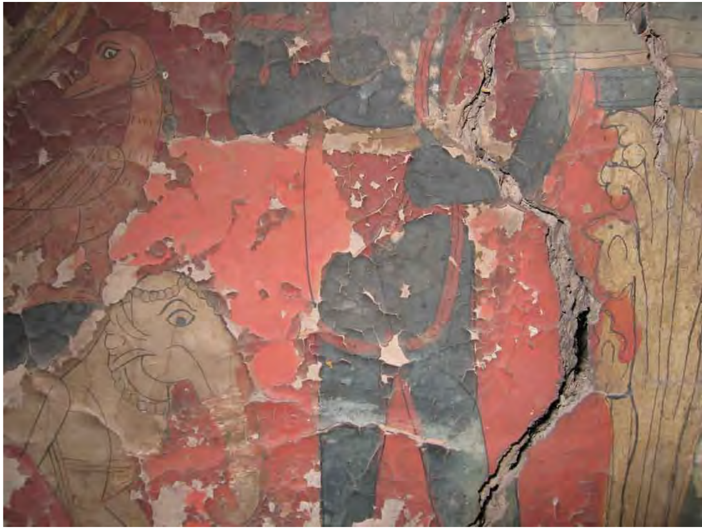
Flaking paintlayer, cracks
