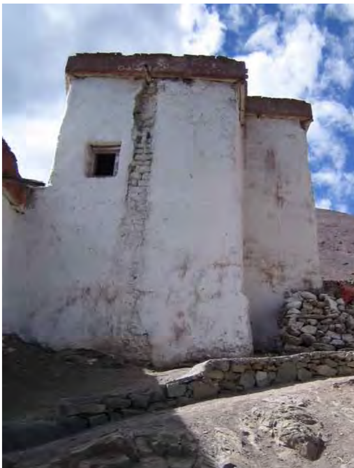
Damaged north wall of Reception room
